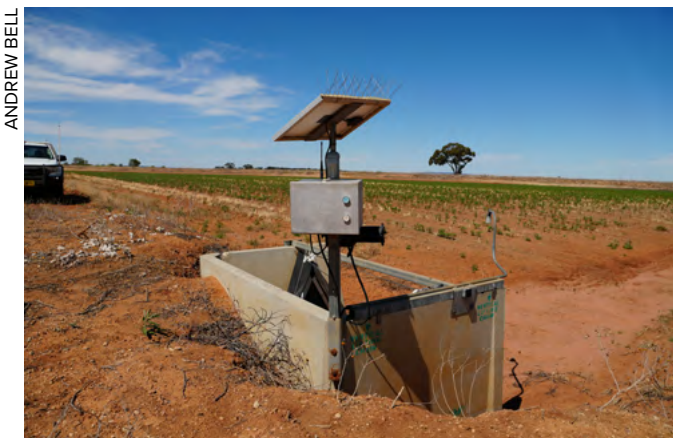
Figure 5: Example of solar powered outlet controller with wired water height sensor and manual override buttons in event of communication failure.
